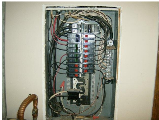
Main Electrical Panel
