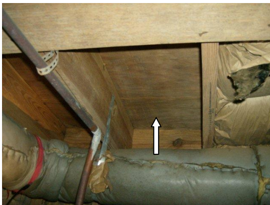
Missing Floor Insulation
