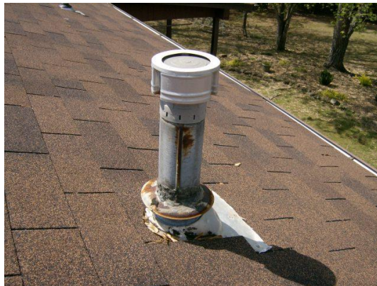
Rusted vent for water heater
