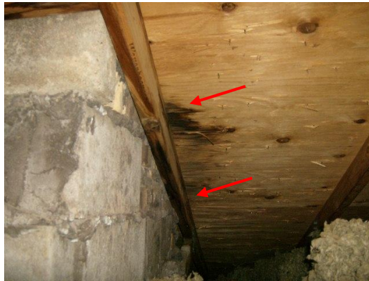
Water Stains near Chimney
